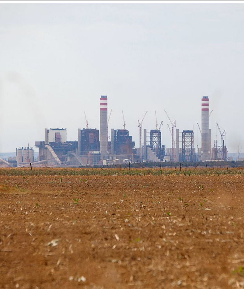
The coal-fired Kusile power plant in eMalahleni (previously Witbank) in the Mpumalanga region
