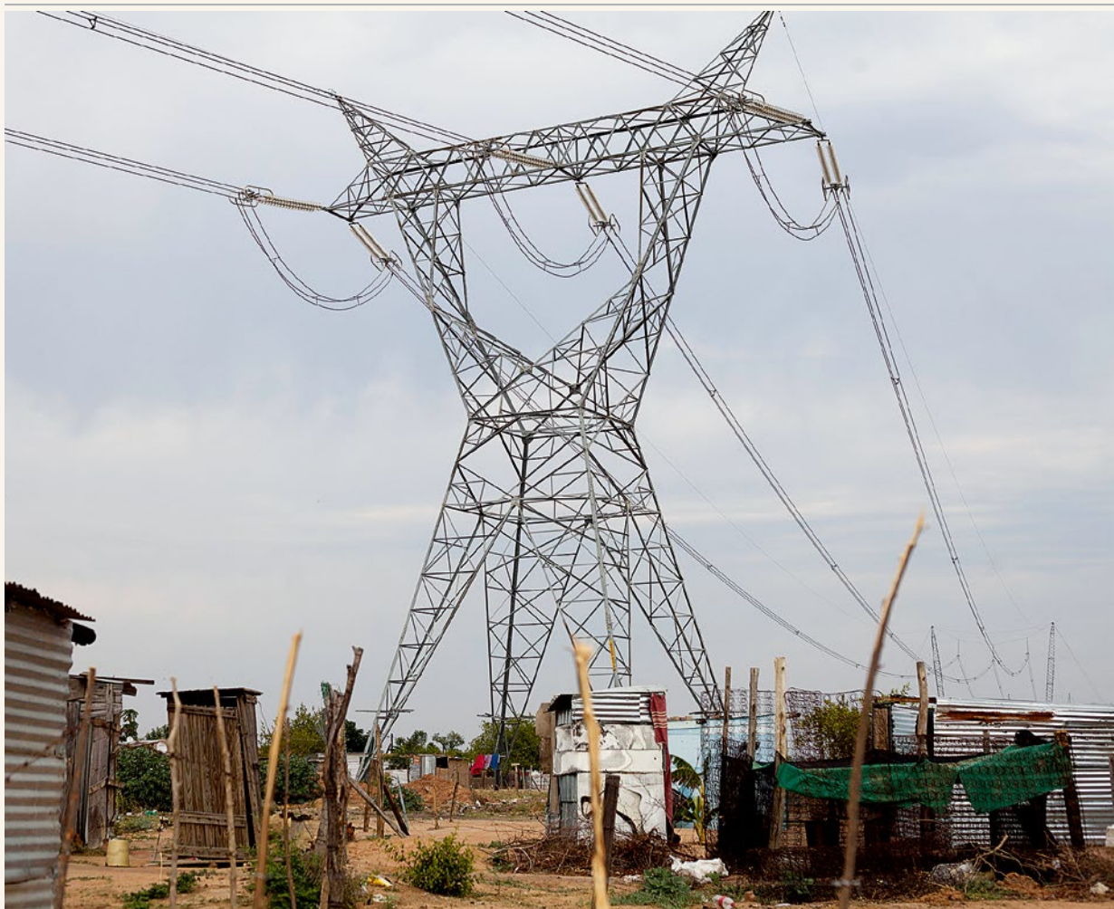
Long power lines run above the shacks of informal settlements. One of the largest power plants is nearby and yet local people have no electricity supply.
