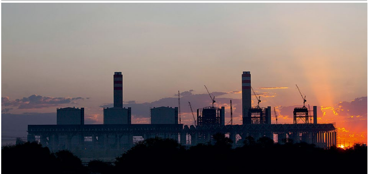
A deceptively romantic scene at the Medupi power plant in Lephalale, Limpopo.
