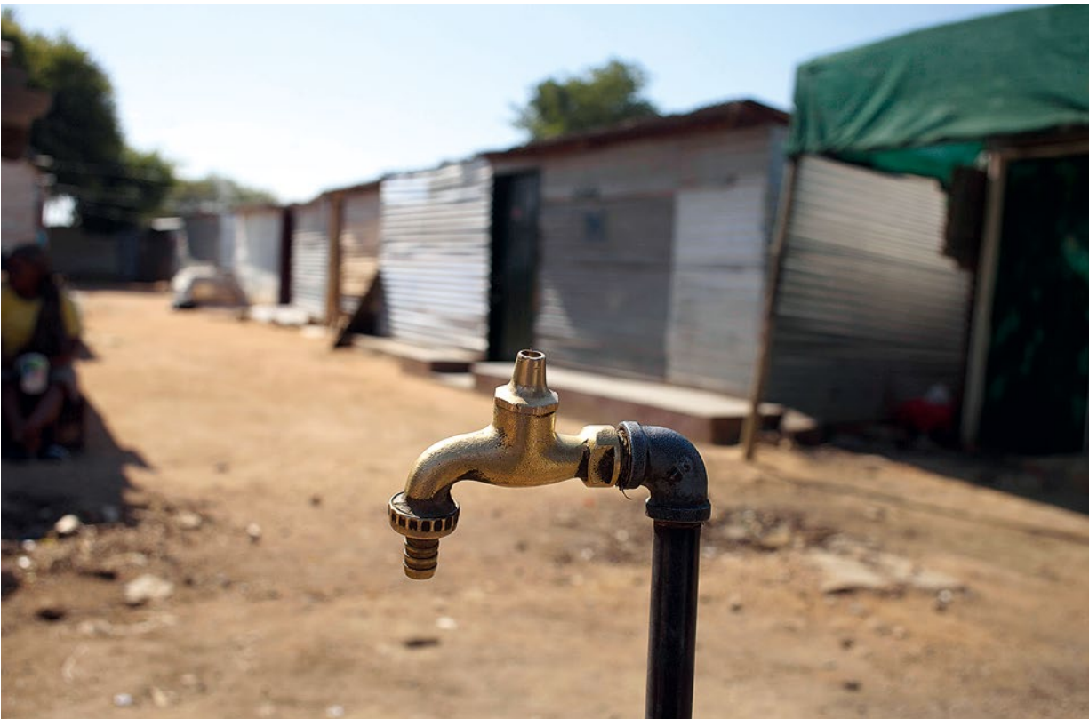
Many inhabitants of the informal settlements have no piped water in their homes. They share public water taps, which are often dry.
